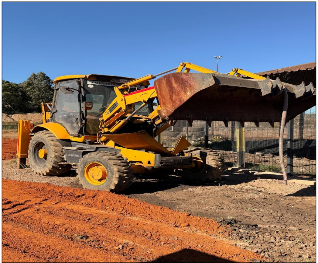
FIGURE 15: TLB and Dozer.(are not working and must be removed from the site.)
