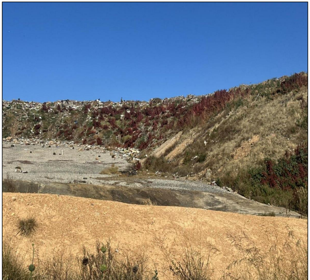
Figure 12: Slope and litter falling onto the new cell development
