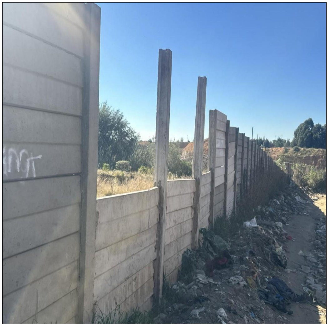
FIGURE 8 Palisade wall damaged
